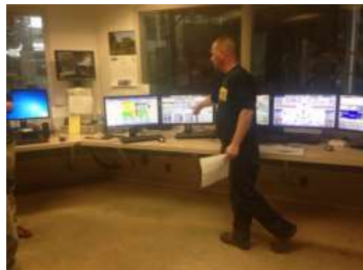
Scott Watkins, KSU Energy Management Supervisor, explains a portion of the CHP control System
